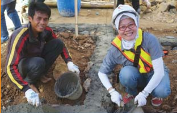
Despite the scorching sun, Rita Tuhali, Ready-mixed concrete Telesales Officer, works enthusiastically on the ground floor structure of a Habitat for Humanity house as part of “Together for Communities” event in July.
